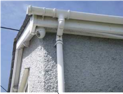
Loose trim to soffit noted, also leaking downpipe joint.
